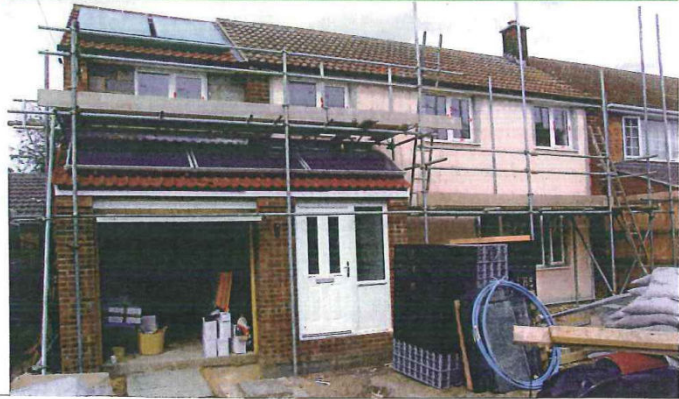
One of two properties acquired by Huntingdonshire District Council as part of BRE's Rethinking Refurbishment project
